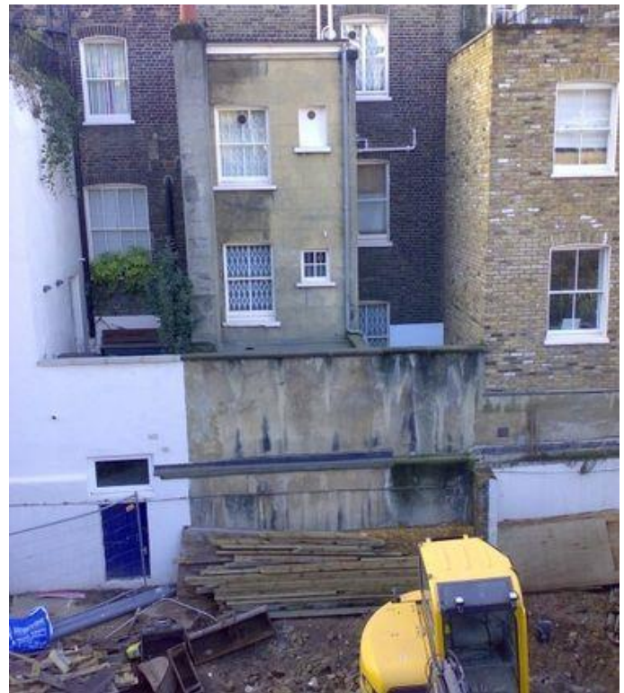
Fig. 1: The basement was to be excavated in very close proximity to sensitive Georgian properties in a congested central London site. (Courtesy: RJM Ground Solutions Ltd)
